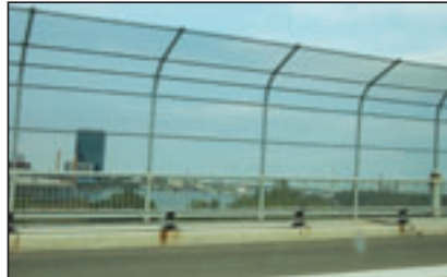
Protective fencing at High Level Bridge extends only over land and not Maumee River despite deaths.
